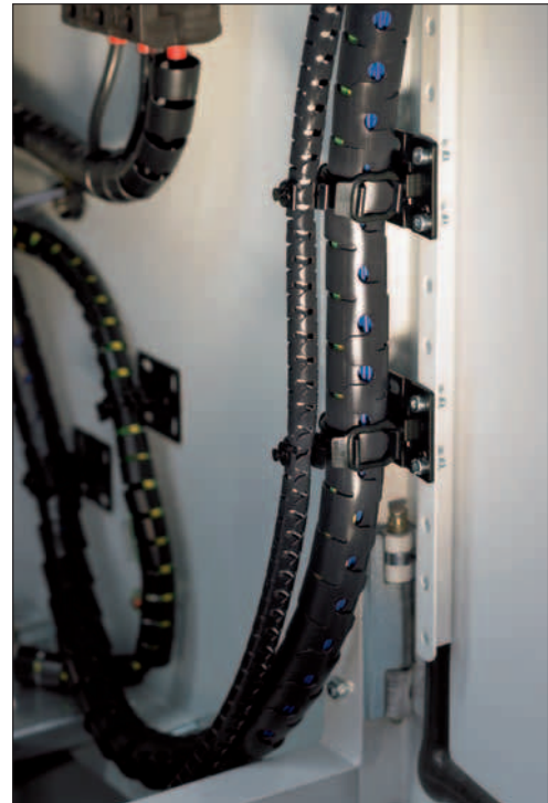
Protecting, fixing and bundling cables with the Helawrap cable cover and accessory set, e.g. in wiring cabinets.
